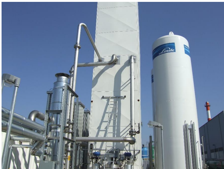
Figure 6: A cold box at a Linde industrial gas facility Source: Linde [55]
