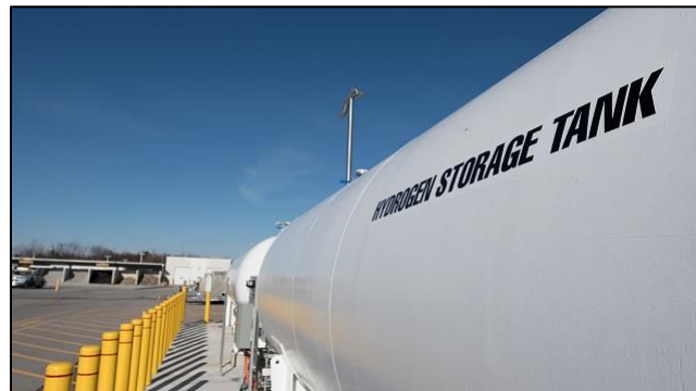
Figure 32: Hydrogen Storage Tank Source: Enbridge Gas [59]
